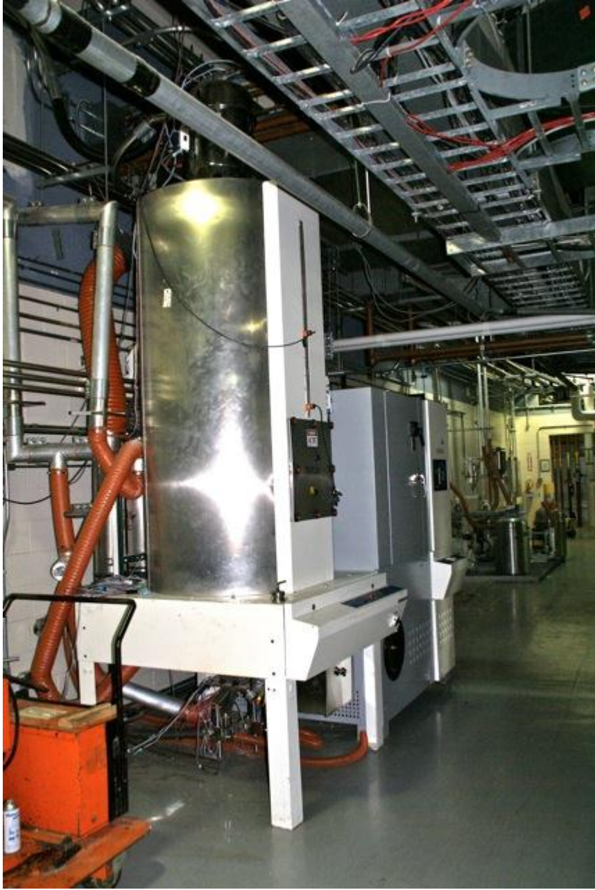
2500 lb Metrolink drying bin
