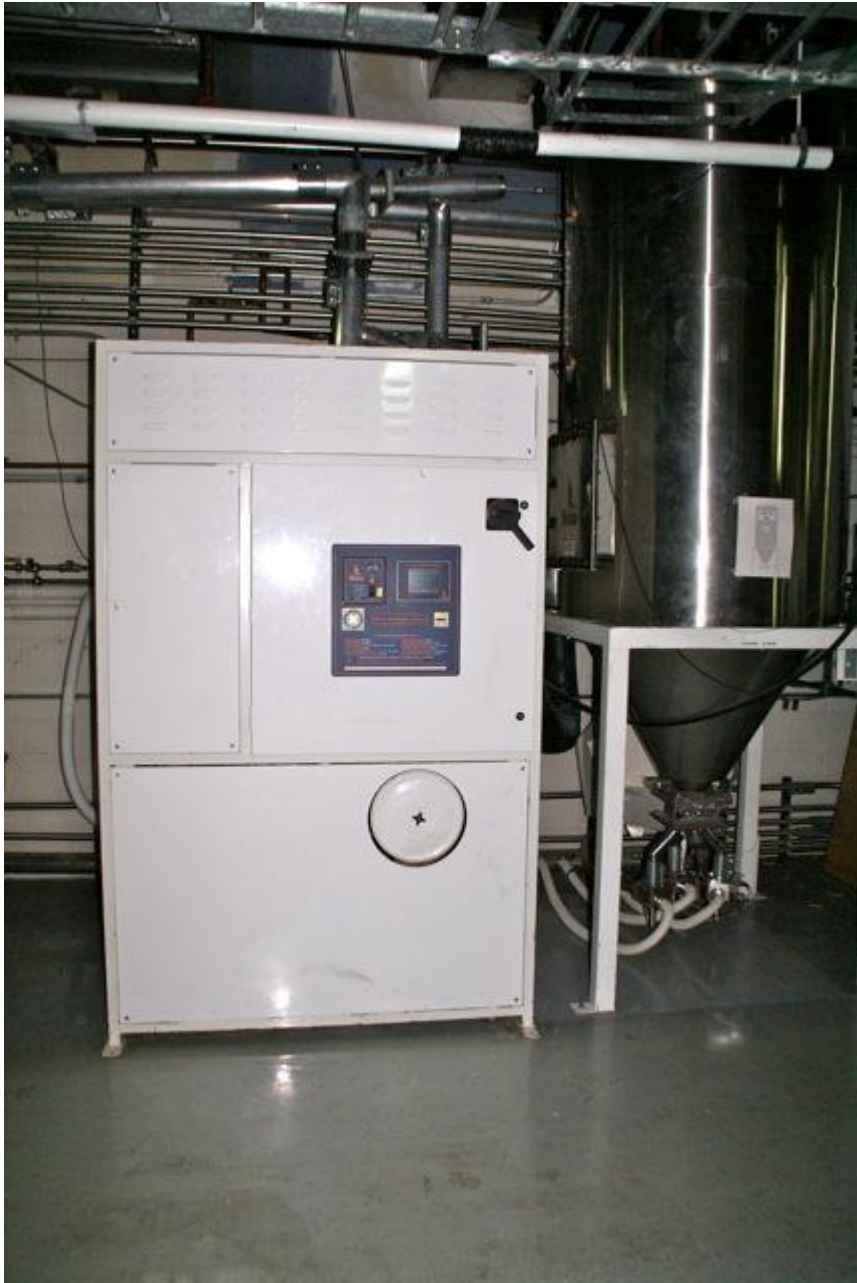
Motan dryer with 3000 lb drying bin
