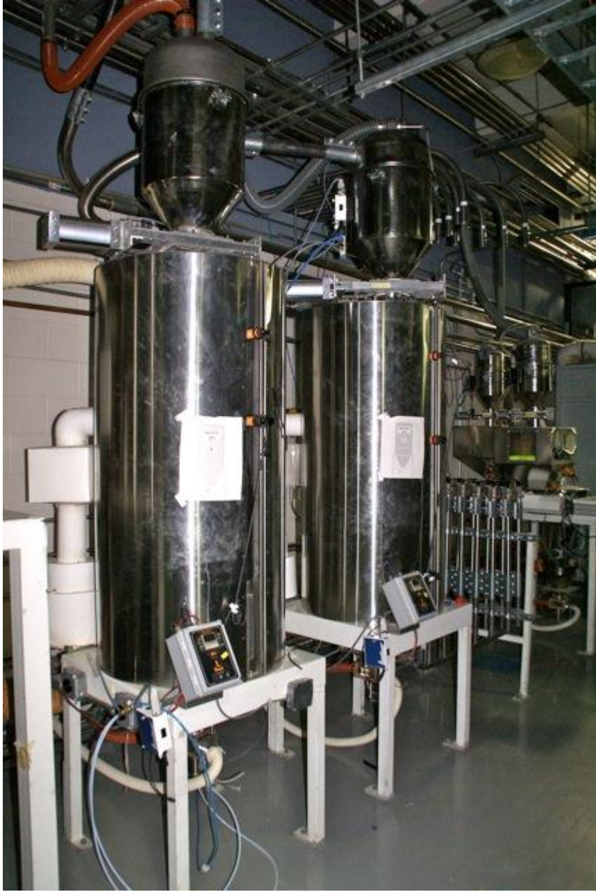
Two (2) 600 lb drying bins associated with two (2) compound blender
