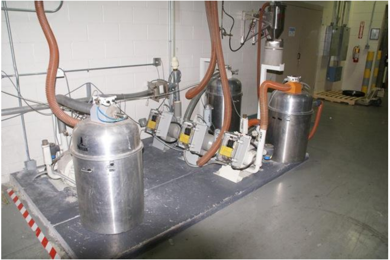
Four (4) 3.4 hp vacuum blowers with three pulse filter fines collectors
