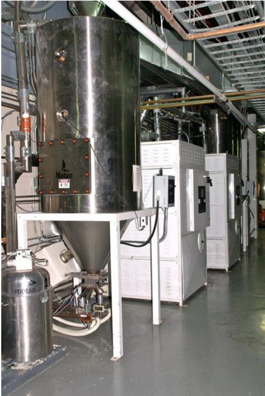
3000 lb Motan drying bin with two (2) Motan dryers
