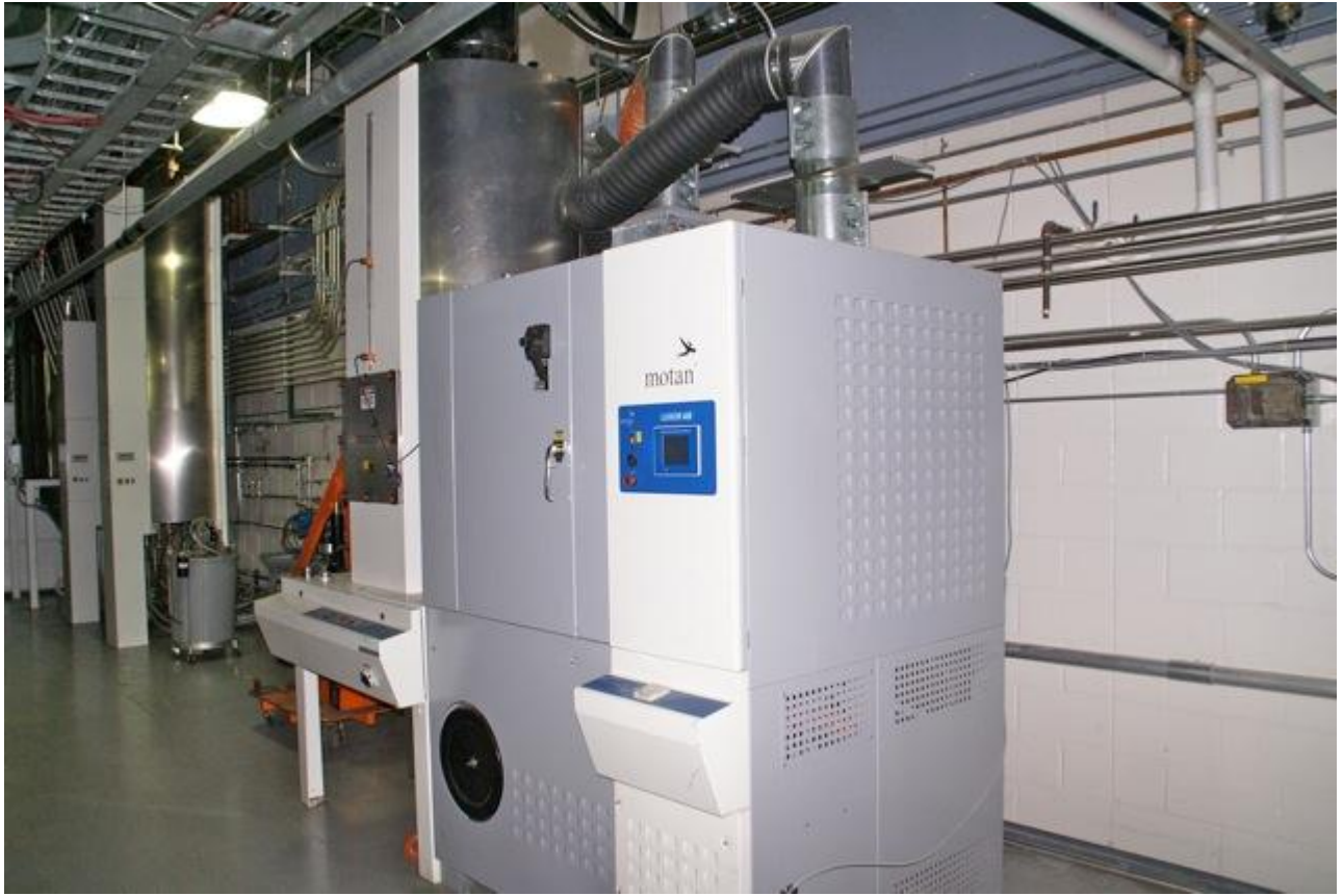
Metrolink Luxor 1600 lb drying bin with control panel and Metrolink Distribution system
