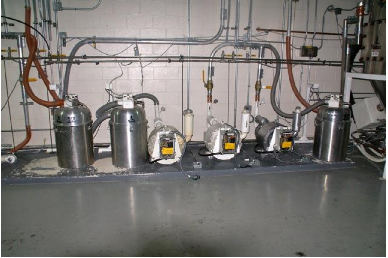
Three 17 hp vacuum blowers with pulse filter fines collectors
