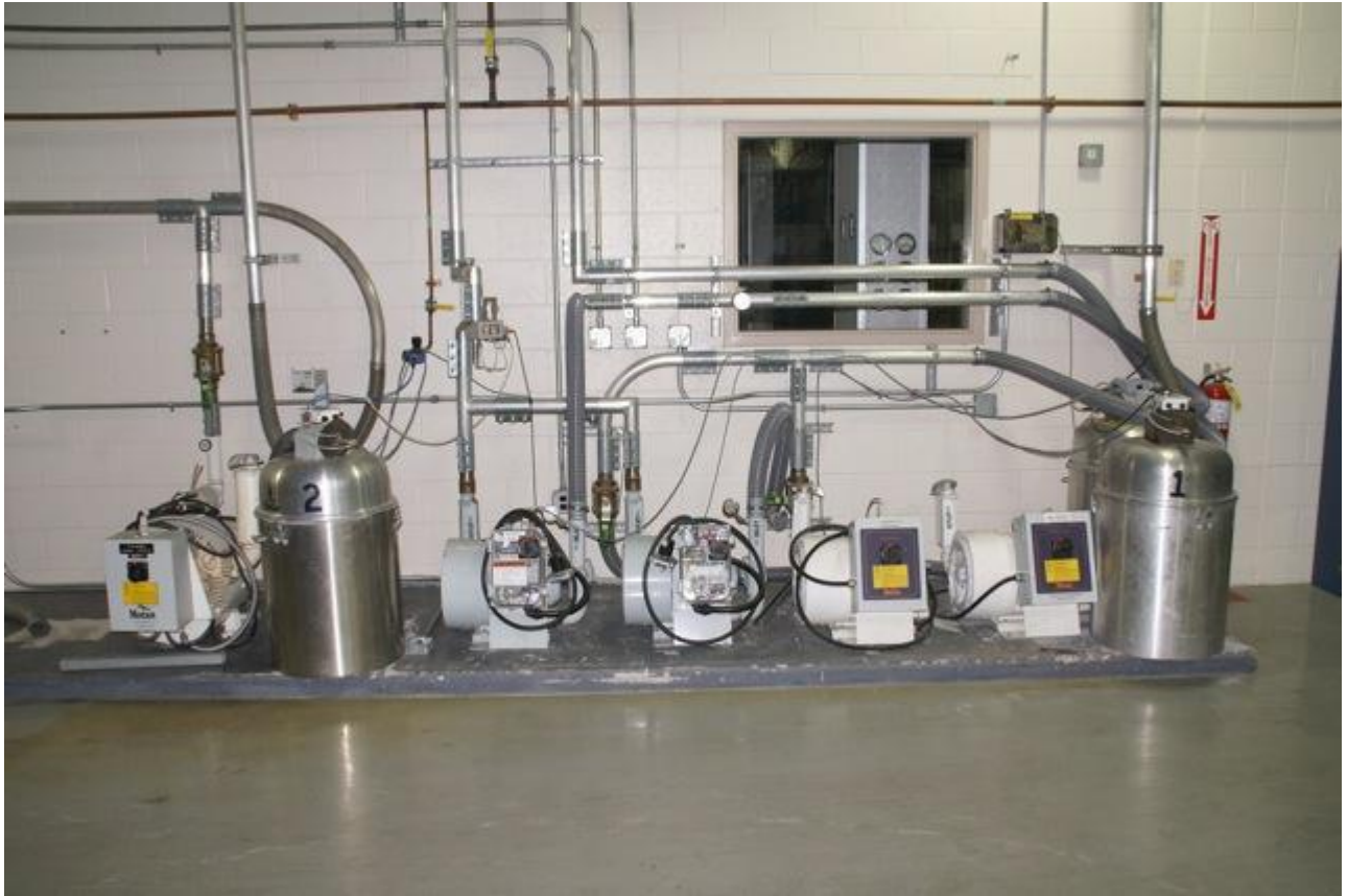
One (1) seventeen hp and four (4) 6.2 hp vacuum blowers with three (3) aluminum pulse filter fines collectors.
