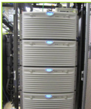
NORTEL NETWORKS MG1000 COMMUNICATION SERVER
