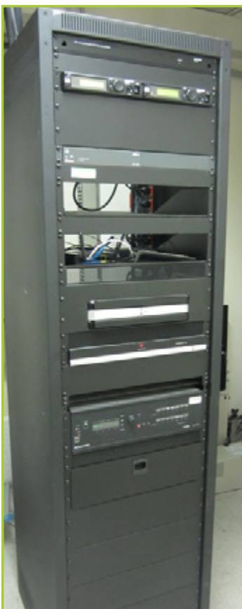
POLYCOM SOUND STRUCTURE C 16, POLYCOM HDX8000 VIDEO CONFERCING SYSTEM
