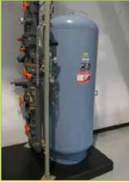
BELL AND GOSSETT EXPANSION TANK
