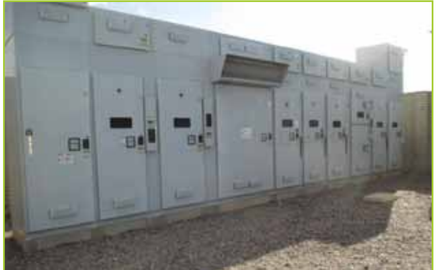
S&C ELECTRIC PUREWAVE PQ2000 SITE UPS, (7) STATIONS, CAPACITY - 12 MW, VOLTAGE - 12,470, BACKUP DURATION - 30 SEC, RECHARGE TIME - 2 MIN FOR EVERY 1 SEC OF DISCHARGE, TRANSFER TIME - 3 MSEC
