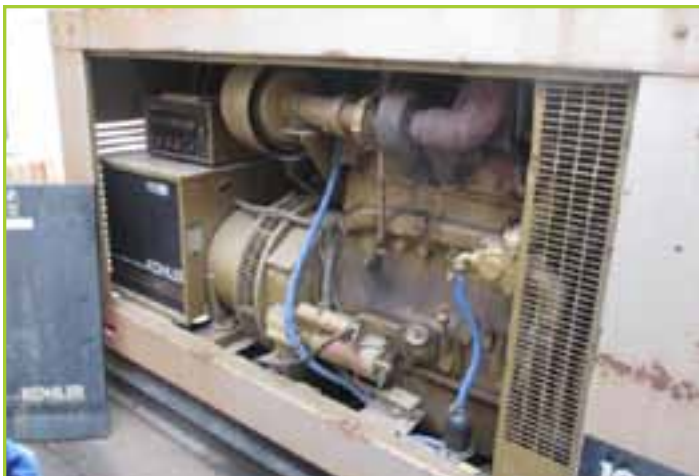
CUMMINGS/KOHLER NT-495-G CUMMINGS 100KW DIESEL GENERATOR , ENGINE HOURS 563, 150 GAL TANK, S/N 25140231, KOHLER MODEL 100R0Z271 S/N 168502
