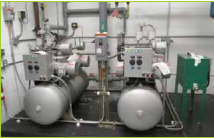
BUSCH RC0100E.506.1003 VACUUM SYSTEM, (2) TYPE R5, ROTARY VANE PUMPS, 63 CFM @ 15 TORR, (2) 5 HP TOSHIBA PUMPS PER TANK, S/N 105373, WITH MOTIVAIR .AC0100 AIR CHILL UNIT
