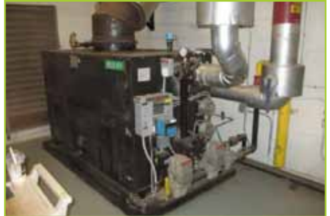
PARKER T2600 NATURAL GAS HOT WATER BOILER, MAX WORKING PRESSURE 150 PSI, HEATING SURFACE 337 SQFT, MAX STEAMING CAP WATER 2080 LB/HR OR MBH, BUILT 95 INSERT YR 2000
