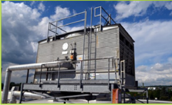
BAC BALTIMORE AIRCOIL ROOFTOP COOLING TOWER, MODEL 3341-LCR
