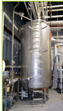
TANK, APPROXIMATE 1750 GALLON
