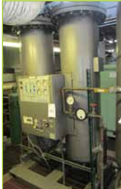
PNEUMATIC 80 NITROGEN GENERATOR
