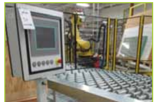
PLC SAFETY SWITCH CONTROLLER CABINET (CABINET FOOTPRINT 7'LX7'HX2'DEEP). INCLUDES: ALLEN BRADLEY LOGIX5563S/ LOGIX55SLP PLC SYSTEM ; AB KINETIX-6500/6000 ETHERNET/ IP-ENABLED SERVO DRIVER SYSTEM ; AB STRATIX8000 ETHERNET MANAGED SWITCH SYSTEM; ASSORTED AB RELAYS; QTY-1 AB PANELVIEWPLUS-1500 TOUCHSCREEN TERMINAL STATIONS
