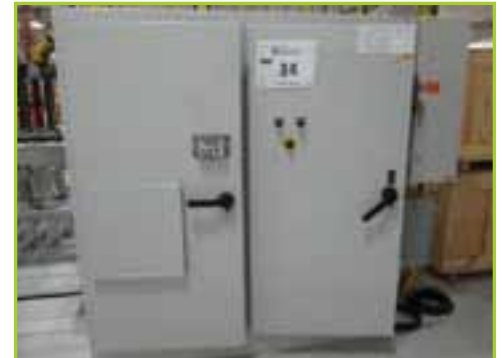
PLC SAFETY SWITCH CONTROLLER CABINET (CABINET FOOTPRINT 7'LX7'HX2'DEEP)
