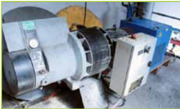
COMPAIR HYDROVANE 43 POWER: 7,5 KW. TOTAL HOURS: 41,680 HR. WITH MTA E800 DRYER AND AIR RECEIVER
