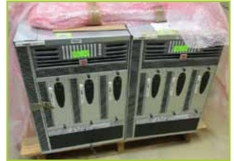
BROCADE 80020207610 SILKWORM 48000 FIBRE CHANNEL (2) SAN SWITCHES
