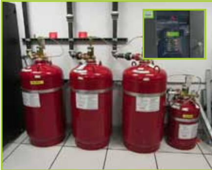
CHEMETRON FM200 FIRE SUPPRESSION SYSTEM
