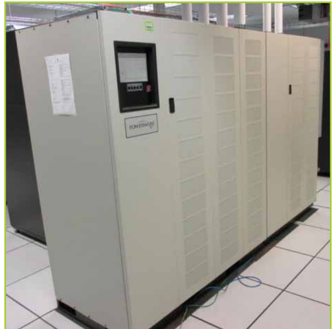
EATON/POWERWARE 9315-300 225 PWHR12390W4FR KVA300, KW240, UPS SYSTEM BATTERIES, 2 STRINGS, 10 TRAYS, 4 JARS
