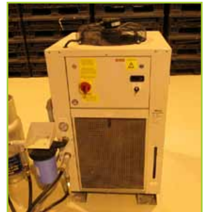
KOOLANT KOOLERS SV2000-W CHILLER, YEAR: 2010
