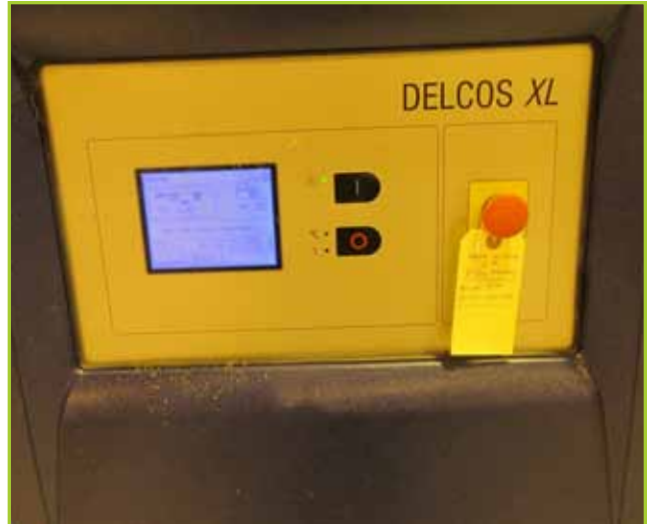
COMPAIR L37RS-13A SCREW TYPE AIR COMPRESSOR , 37 KW MOTOR, 460V, 3 PHASE, 60HZ, DELCOS XL CONTROLS. SN# CD10005426001. YEAR: 2011
