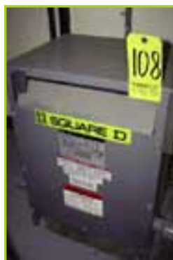
SQUARE D TRANSFORMER
