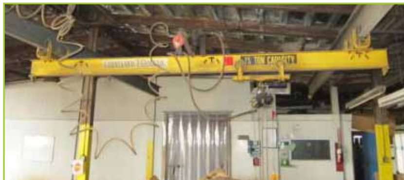
APPROXIMATELY 14' SPAN UNDER RUNNING BRIDGE CRANE WITH PNEUMATIC HOIST
