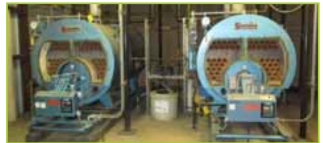
CONTENTS OF BOILER ROOM TO INCLUDE (2) SUPERIOR BOILER WORKS BOILERS, INDUSTRIAL STEAM FEED WATER SYSTEM, SPILL PALLET, STORAGE CABINET WITH CONTENTS, WERNER 8' 300LBS CAPACITY FIBERGLAS LADDER. CHEMICAL STORAGE
