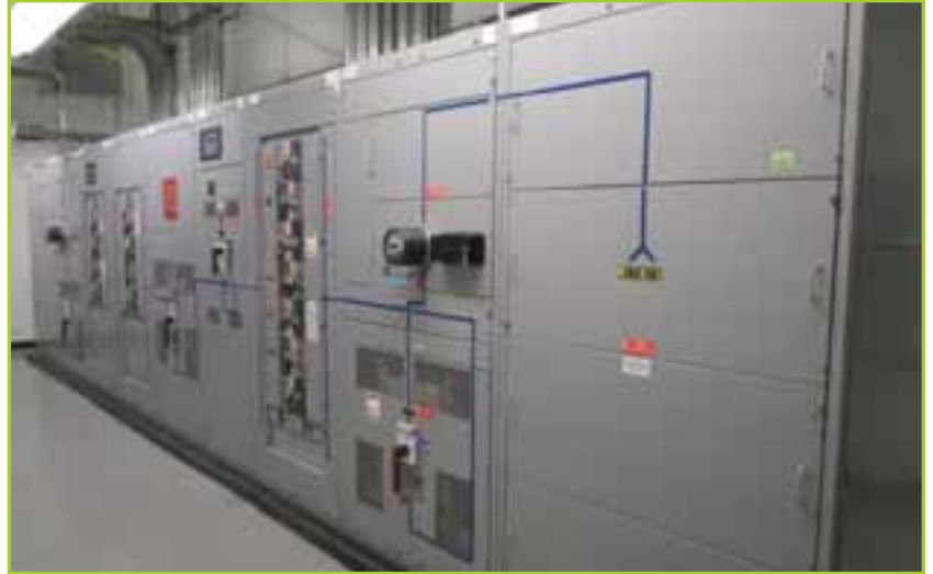
LOT: QTY (2) SWITCHGEAR STATIONS (9) SECTIONS GE SPECTRA SERIES 3000 AMP, (4) GE SPECTRA SERIES POWER PANELS, (8) SECTIONS SQUARE D 74651 I-LINE 2000 AMP
