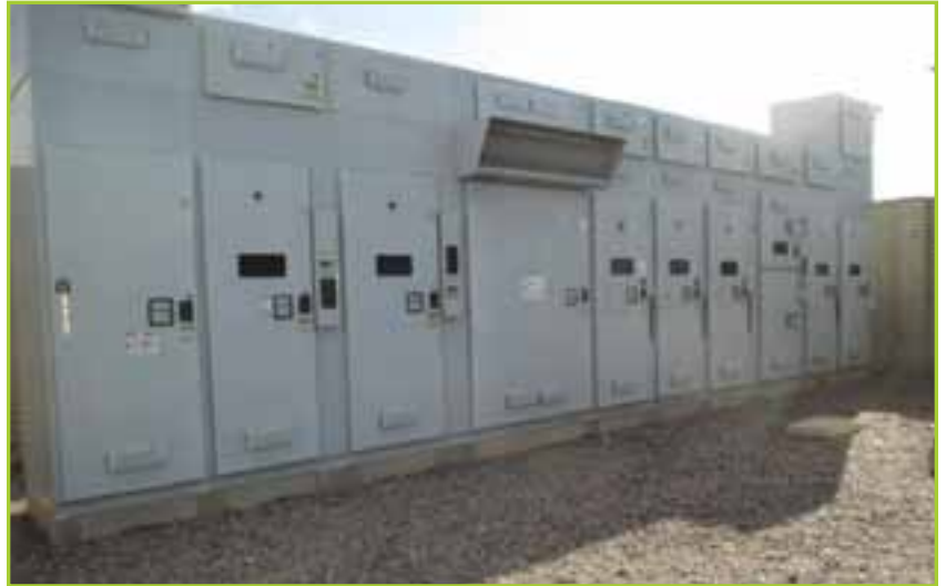
S&C ELECTRIC PUREWAVE PQ2000 SITE UPS, (7) STATIONS, CAPACITY - 12 MW, VOLTAGE - 12,470, BACKUP DURATION - 30 SEC, RECHARGE TIME - 2 MIN FOR EVERY 1 SEC OF DISCHARGE, TRANSFER TIME - 3 MSEC
