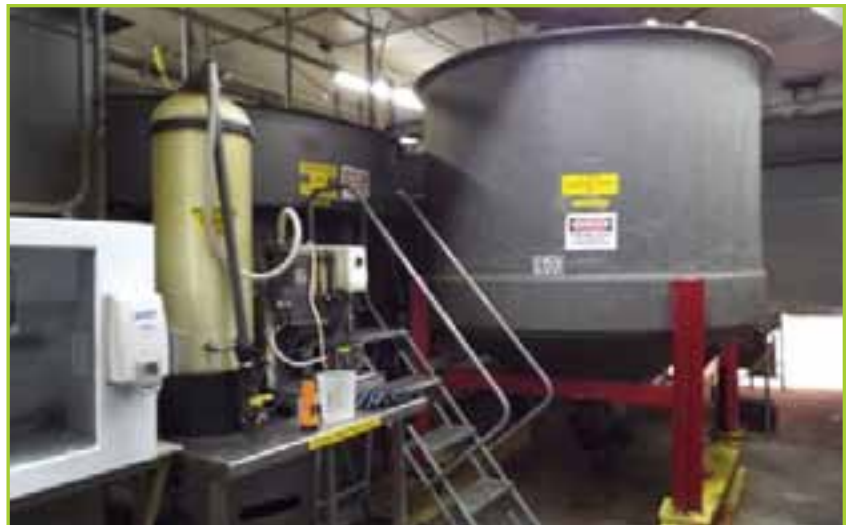
ANDERSON NICKLES DAF WASTE WATER TREATMENT SYSTEM INCLUDES 45,000 GALLON EQUALIZATION TANK, (2) 11,000 BIO TANKS, DAF UNIT, TRANSFER PUMPS, ROTO STRAINER, WASTE SCREW CONVEYOR AND SLUDGE CONTAINER
