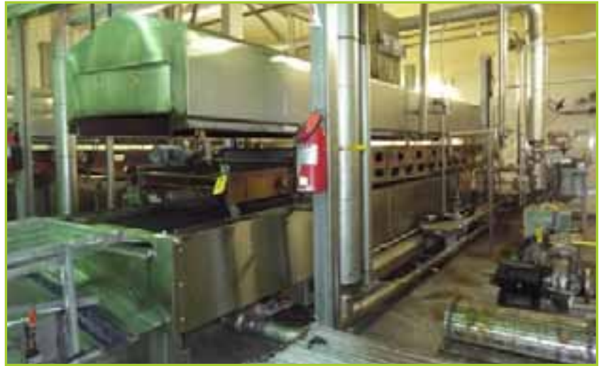
HEAT & CONTROL FRYER, MODEL BPF, PROJECT# 2003004520, 460 VOLTS, 6.6 AMPS, 3 PHASE 60 HZ, WITH CORNELL DUMP, FILTER, HEXCHANGER & HOLD TANK, 37 IN. BELT, 28 FT. LONG
