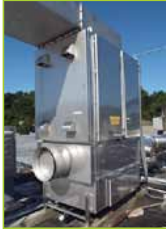
JIMCO AIR CLEANING SYSTEM CONSISTS OF SS ENCLOSURE WITH (60) 180W UV LAMPS
