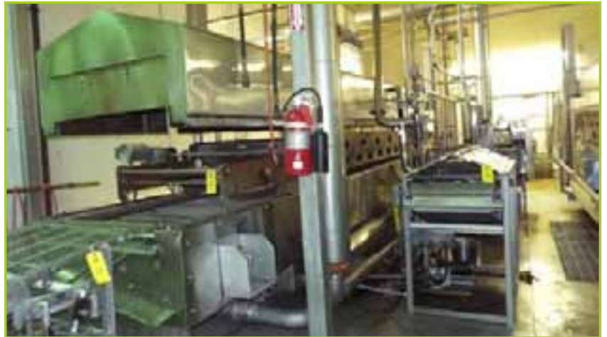
HEAT & CONTROL FRYER, MODEL BPF, PROJECT# 2003004520, 460 VOLTS, 6.6 AMPS, 3 PHASE 60 HZ, WITH CORNELL DUMP, FILTER, HEXCHANGER & HOLD TANK, 37 IN. BELT, 28 FT. LONG
