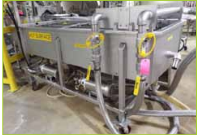
SS DEGLAZING TANK WITH 2 WASH DOWN MOTORS, 3 DIMPLE PLATES
