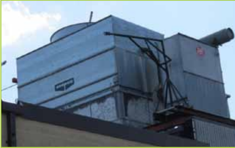
EVAPCO EVAPORATIVE CONDENSER, MODEL:ATC-442B S/N: 8-384012
