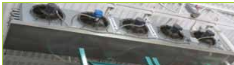
(19) 2006 VILTER AMMONIA BLOWERS
