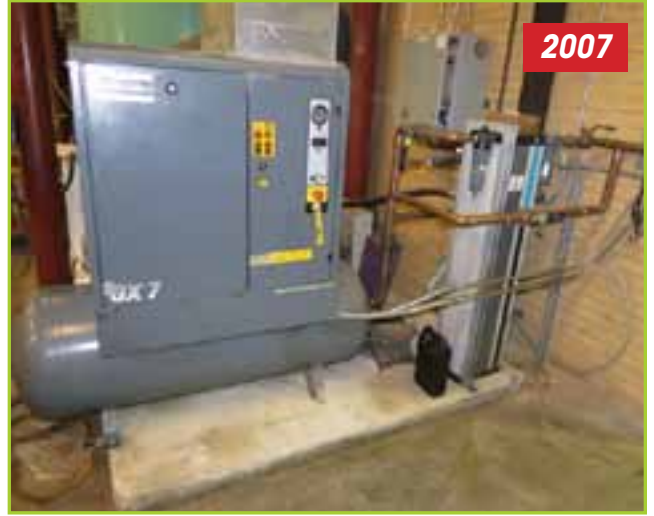
2007 ATLAS COPCO AIR COMPRESSORS
