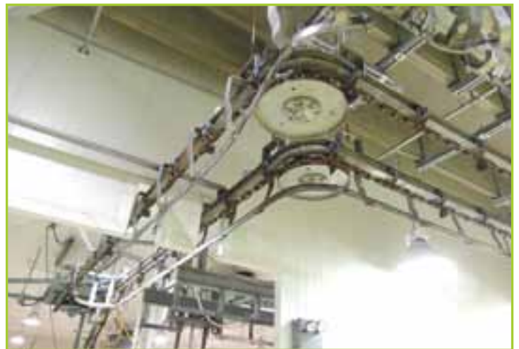
APPROXIMATELY 450' MEAT RAIL SYSTEM, WITH INCLINE, SWITCHES, DRIVE CHAIN, LOWERATOR AND DRIVES
