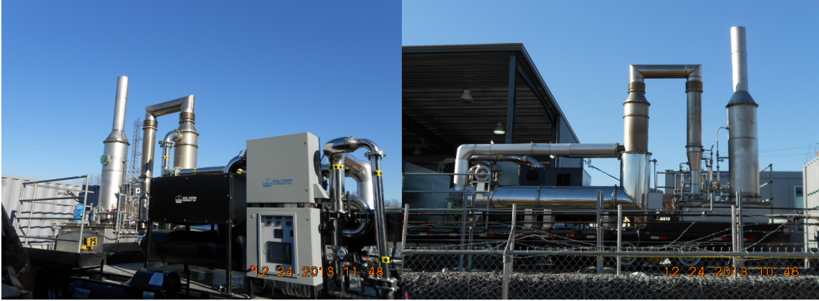
View of Control Panel, Enclosed Blowers View of Heat Exchanger and Scrubber Assembly
