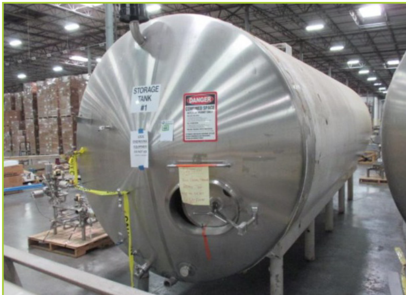
FELDMER A-865-1 5000-GALLON JACKETED TANK (HORIZONTAL; ON LEGS; OVERALL FOOTPRINT 23.5'LX8'WX11'H ; TANK ID#1)
