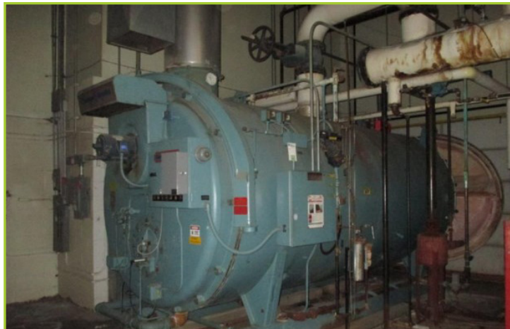
CLEAVER BROOKS CB-200-200 200-HP LOW PRESSURE CB PACKAGED GAS-OIL-FIRED BOILER
