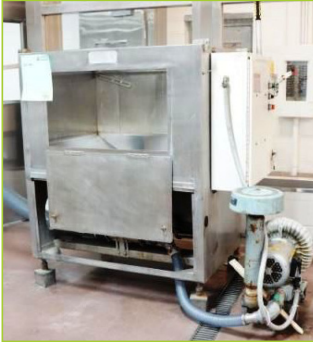
ALCOA JETFLOW CAP BLOWER. GAST 5 HP BLOWER. PIPING TO CAPPER
