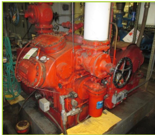
VILTER A446 75-HP 6-CYLINDER AMMONIA COMPRESSOR
