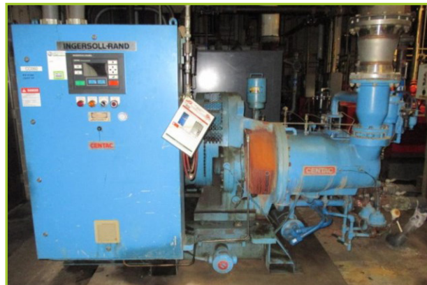
INGERSOLL RAND CENTAC-1CV14M2 400-HP CENTRIFUGAL AIR COMPRESSOR [S/N-M99-10371 ; YEAR 1999. DESIGN: CFM 1852 ; PSIA 14.2 ; PSIG 115 ; RPM 3575. WITH SIEMENS 400-HP INDUCTION MOTOR
