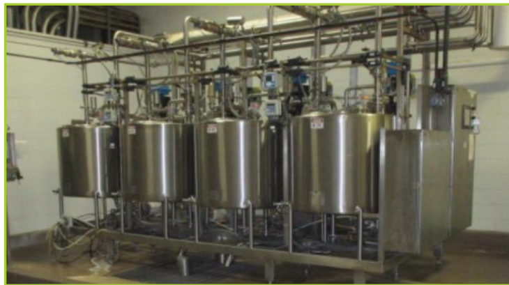
RDM (4-TANK) SANITATION CIP SYSTEM SKID (FOOTPRINT 18'LX9'WX10.5'H ; WITH QTY-2 CONTROL CABINETS) (SYSTEM HAD SERVICED 4 BOTTLE LINE FILLERS). [EACH TANK: 200-GALLON ; BY A&B PROCESS SYSTEMS ; STAINLESS STEEL. #1 MODEL-200CTA S/N-31299301A ; #2 MODEL-200CTC S/N-31299301C ; #3 MODEL-200CTB S/N-31299301B ; #4 MODEL-200CTD S/N-31299301D] [EACH TANK SUPPORTED BY: VIEX PLATE HEAT EXCHANGERS ; ROSEMONT 1056 OR SOLUCOMP-II MULTI-PARAMETER ANALYZER ; WAUKESHA CHERRY-BURRELL 10HP/BALDOR PUMP]
